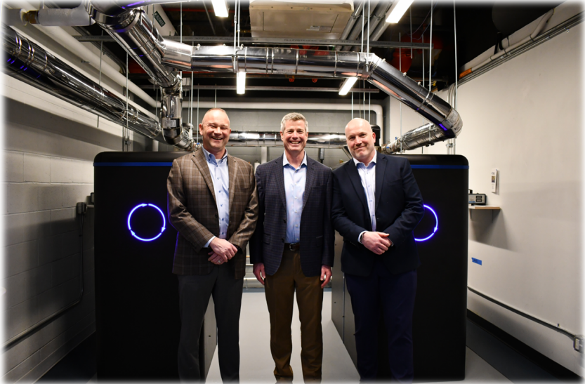
NJR President & CEO Steve Westhoven, NJNG COO Pat Migliaccio and CEO & Founder of Clean02 Jaeson Cardiff standing in front of two operational CarbinX units in the mechanical room of NJNG's Corporate Headquarters
