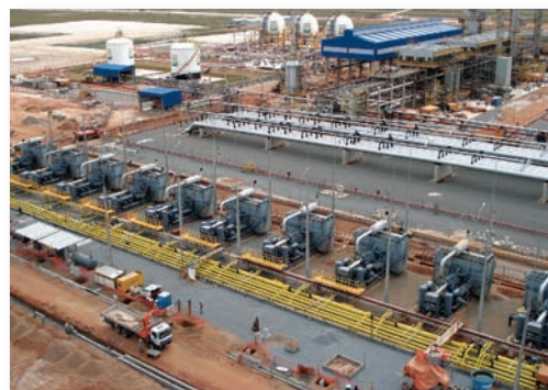
Contract compression units at a production and processing facility in Brazil
