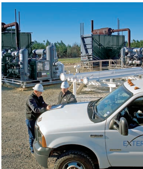
Contract compression operation in East Texas
